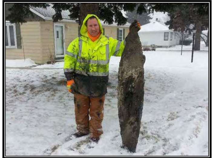
Blow-off from a 16" water main on 47th Avenue
