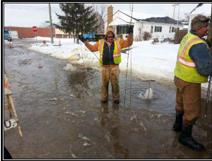
6" main break floods 10th Avenue
