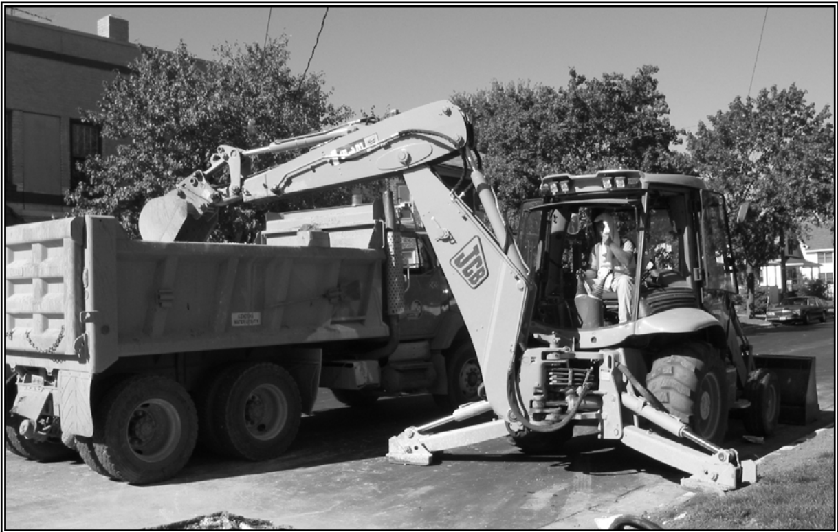
Construction equipment currently used by the Water Distribution and Sewer Collection Division.
