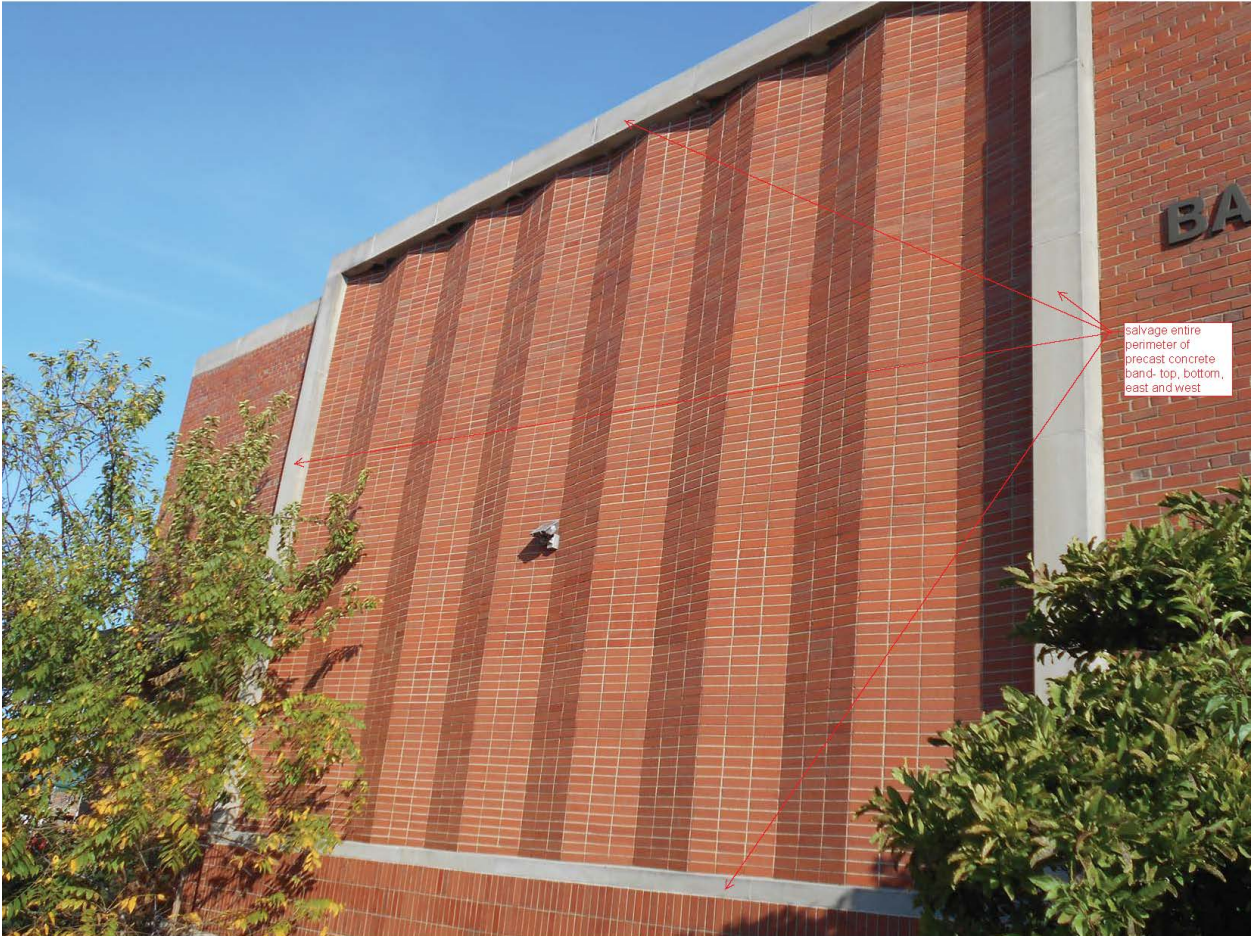
Item 7: The continuous precast frame on the south side of the building. All 4 pieces.
